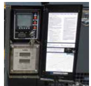
Operator's Control Station
