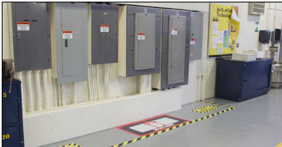
Electrical Panels be marked to notify people they are not to block.
