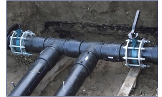
Construction Water Effluent Lines
